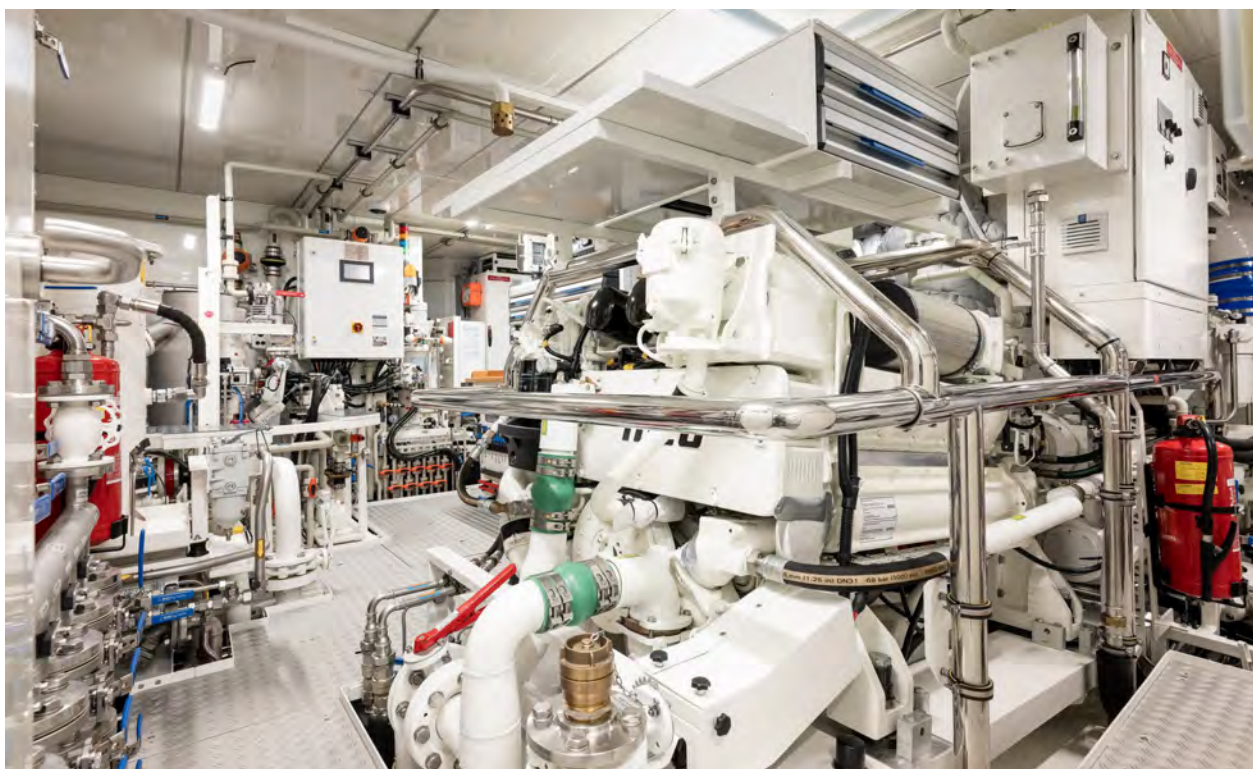
PROVEN SEMI-HYBRID TECHNOLOGIES AND A 134KW BATTERY BANK FOR PEAK SHAVING
